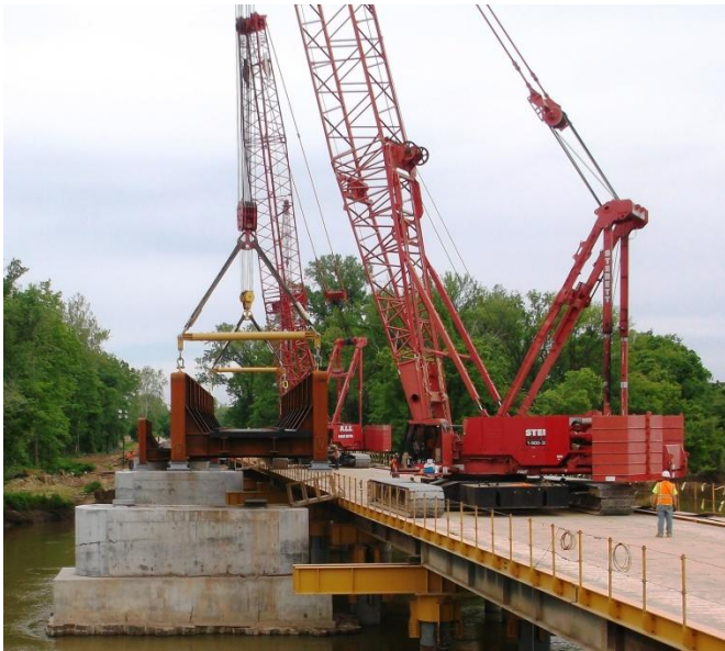
Construction cranes lift the new through plate girder bridge spans into place on rebuilt bridge piers.
