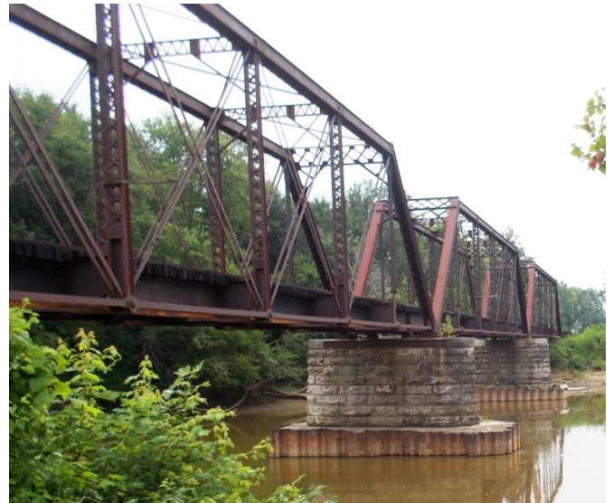
The original White River Freight Railroad Bridge, which opened when William McKinley was president, was functional for 115 years.
