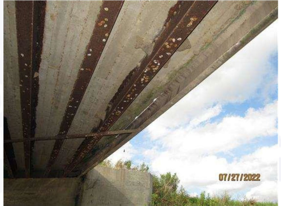
Image taken from inspection report
