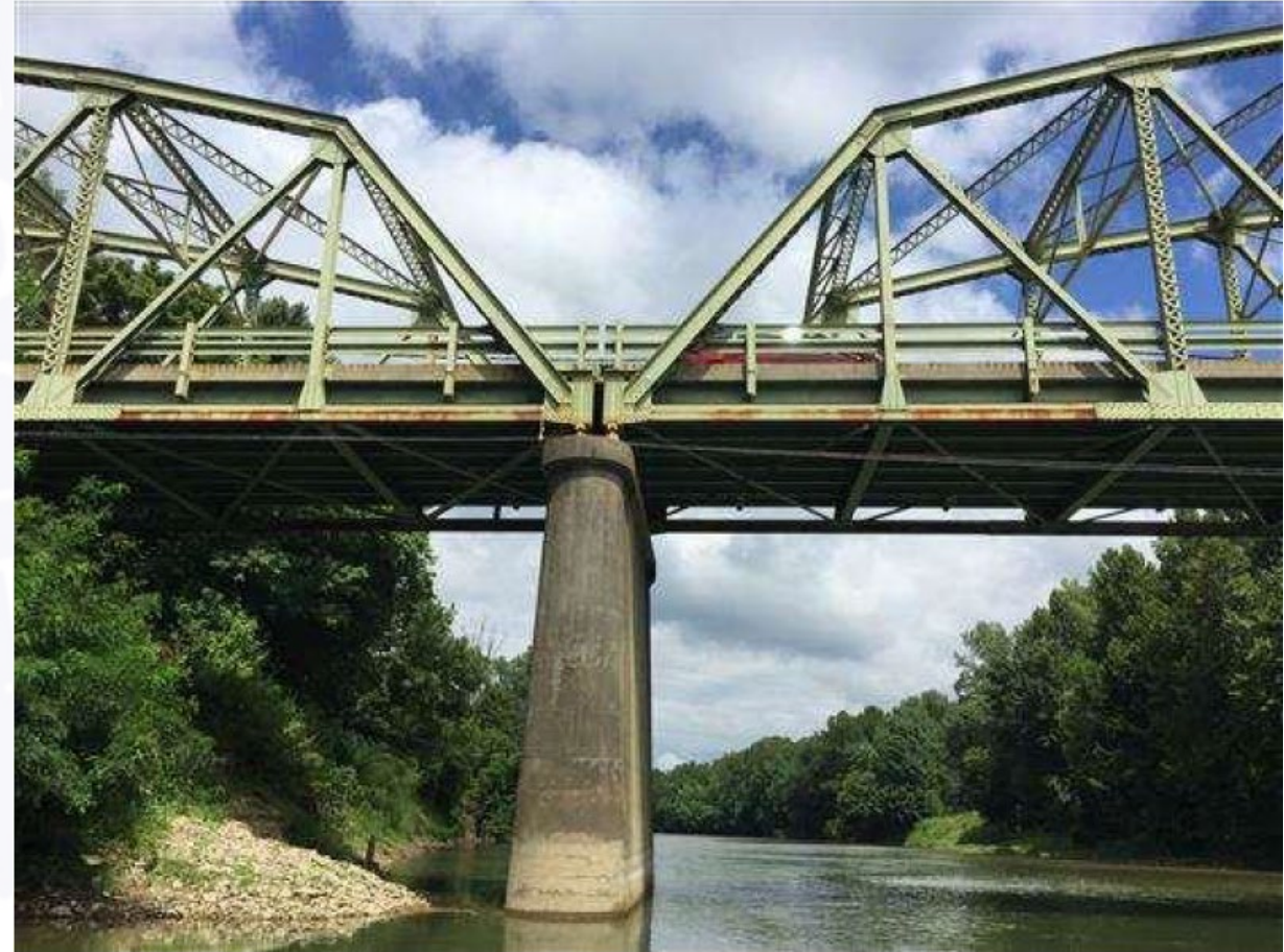
Image taken from inspection report
