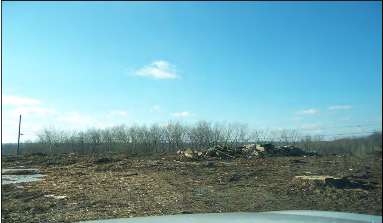
Looking west at the west end of Aretz Lane at recently demolished residences
