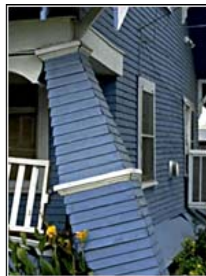
Figure 3-6 Earthquake Damaged Porch
