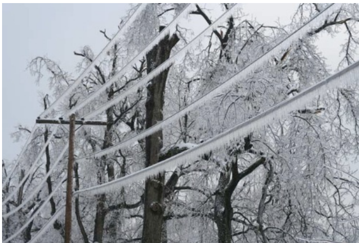
Figure 3-22 Ice Covered Power Lines
