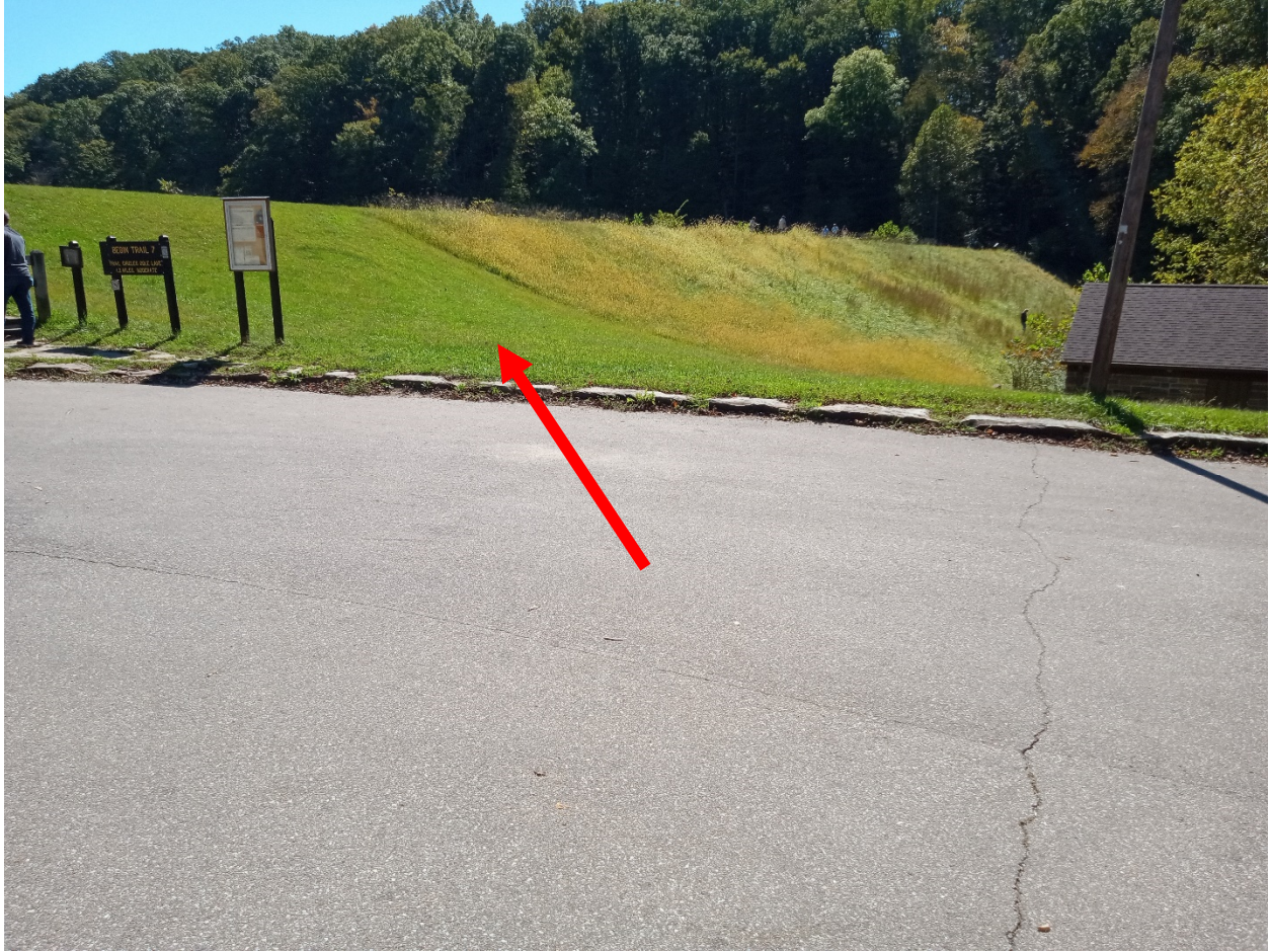
Dam crest access location. Contractor to protect asphalt parking and stone curb. Return back to existing condition.
