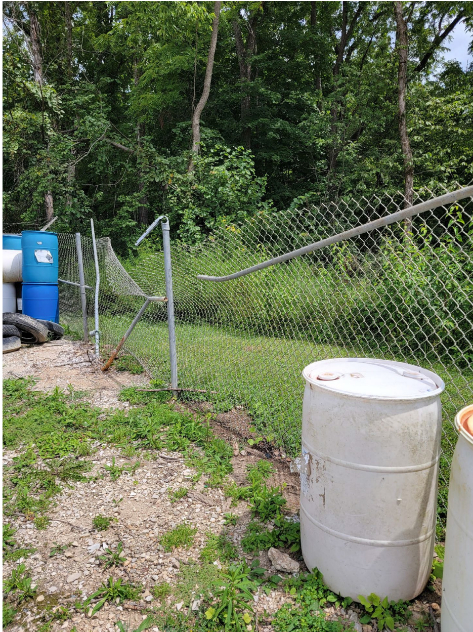
Photograph No. 9 – Existing Fence Damage
