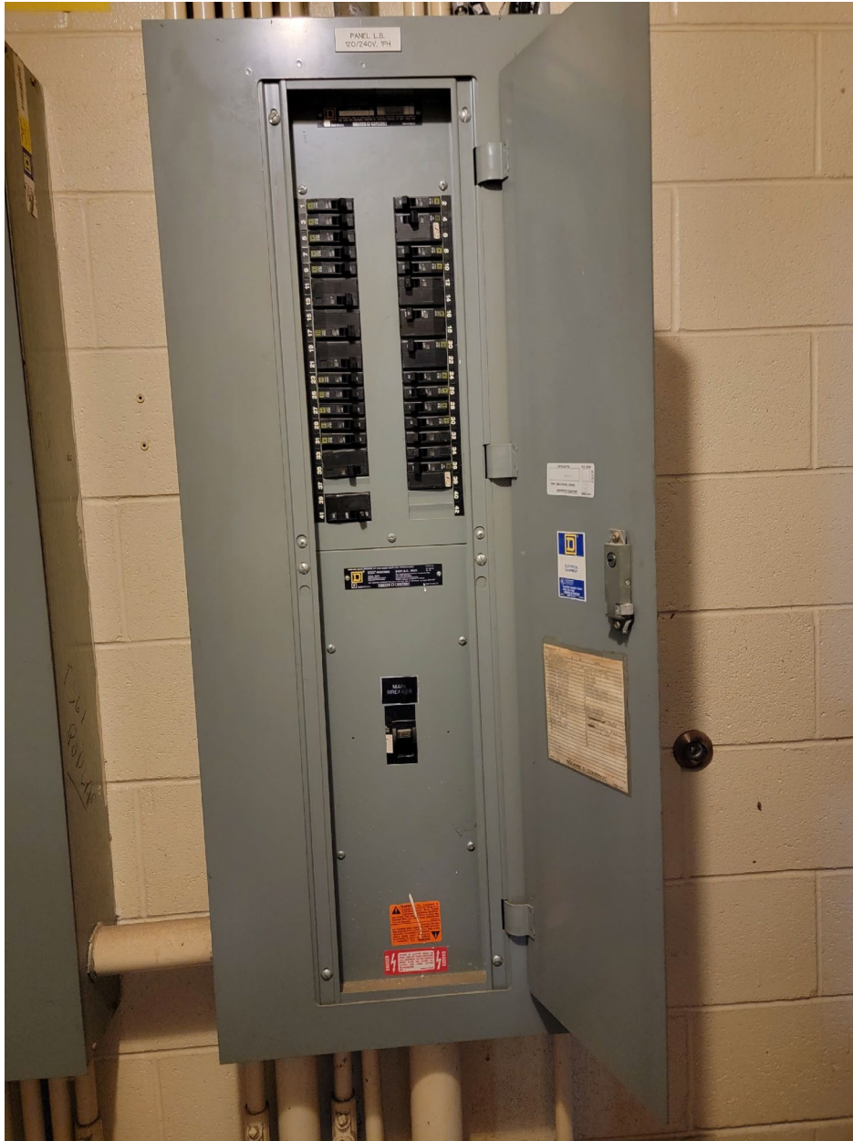
Photograph No. 4 – Existing Maintenance Building – Existing Electrical Panel L.B. 120/240V 1PH
