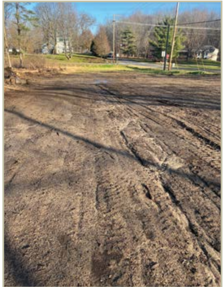
This landing was smoothed well, but not stabilized with seed or straw/mulch and therefore sheet and rill erosion is occurring. Photo by Jennifer Sobecki, DNR
