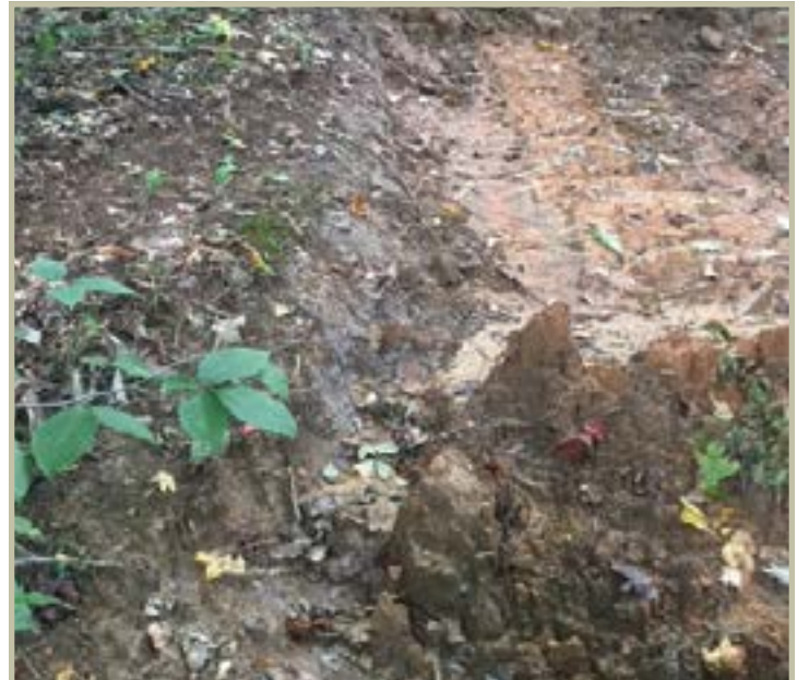
Breach of a waterbar due to lack of outlet. Photo by Jennifer Sobecki, DNR
