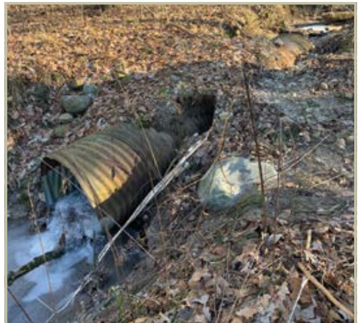
The culvert is too small for this drainage and thus is being washed out. This leads not only to sediment in the streams but dangerous crossing conditions. Photo by Jennifer Sobecki, DNR
