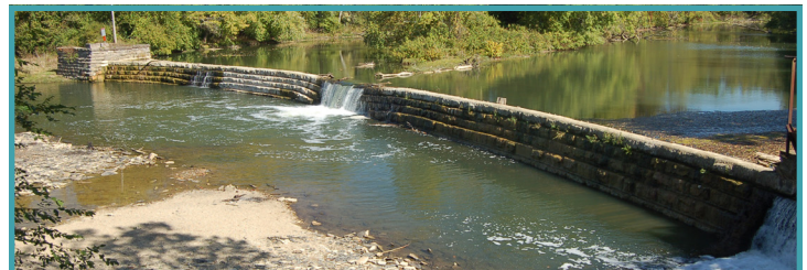
Water cascades through and over the deteriorating Thompson Mill Dam in Edinburgh in autumn 2023.
