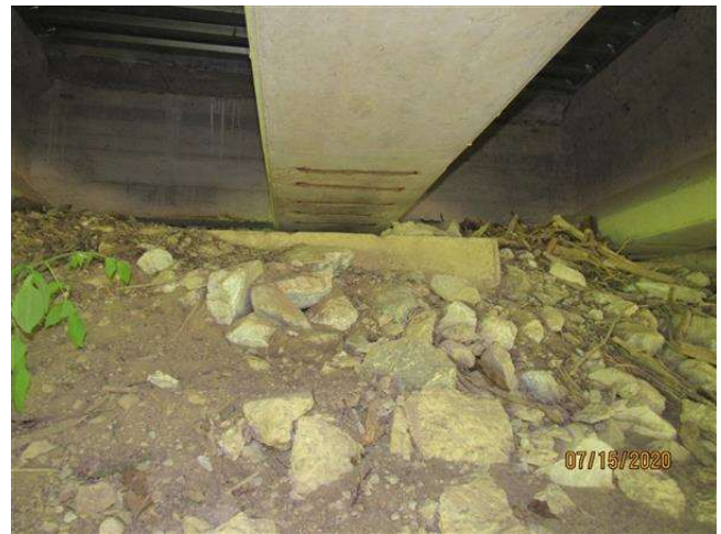
Exposed Straps at Beam 3 End
