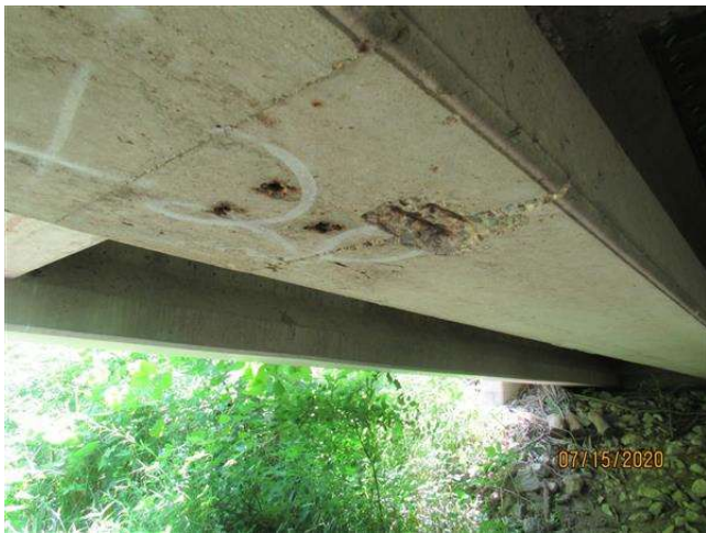
Exposed Steel Bars in Beam 2
