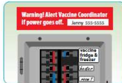
Label fuses and circuit breakers. Post a sign to alert the Vaccine Coordinator any time the power goes out.
