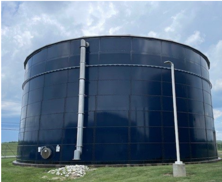
Figure 4.2 – Ground Level Storage Tank
