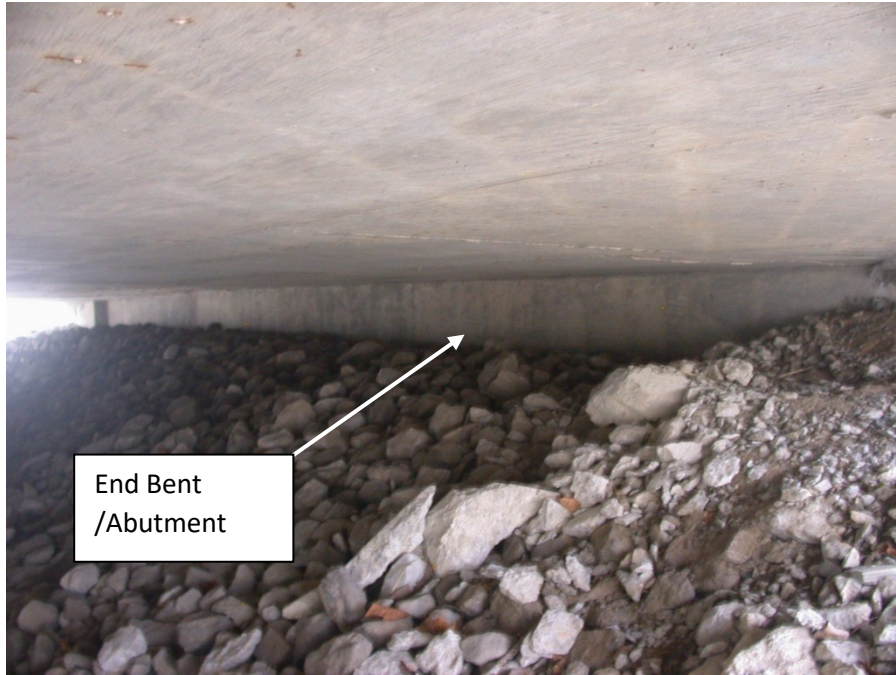
Underside of this Reinforced Concrete Slab Bridge at end bent/abutment, no bridge seats, bearing assemblies, beam/girder ends, or mudwalls to clean or flush.
