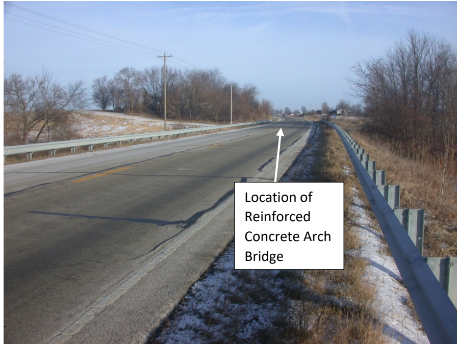
Reinforced Concrete Arch Bridge (Under Fill) with no bridge railings, curbs, or bridge deck expansion joints so no cleaning or flushing activities required.
