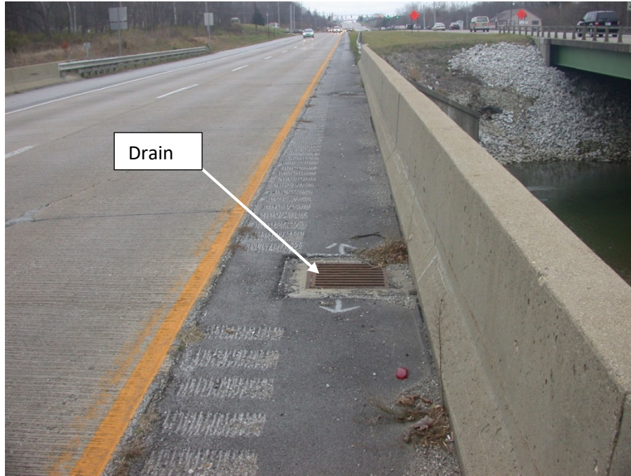
Drain in Reinforced Concrete Arch Bridge, cleaning and flushing required. (Activity 2410)
