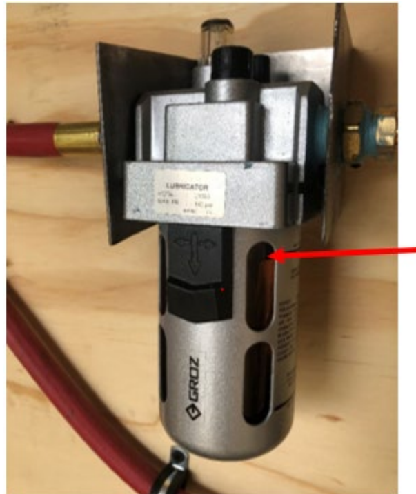
Figure 5: Oil level in lift pump container
