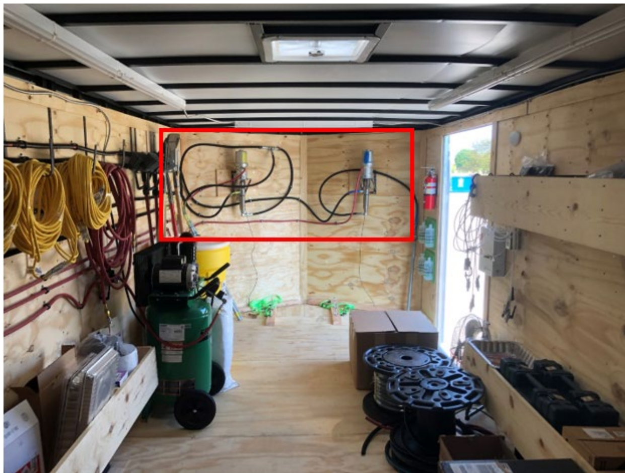
Figure 3: Location of lift pumps and oil containers
