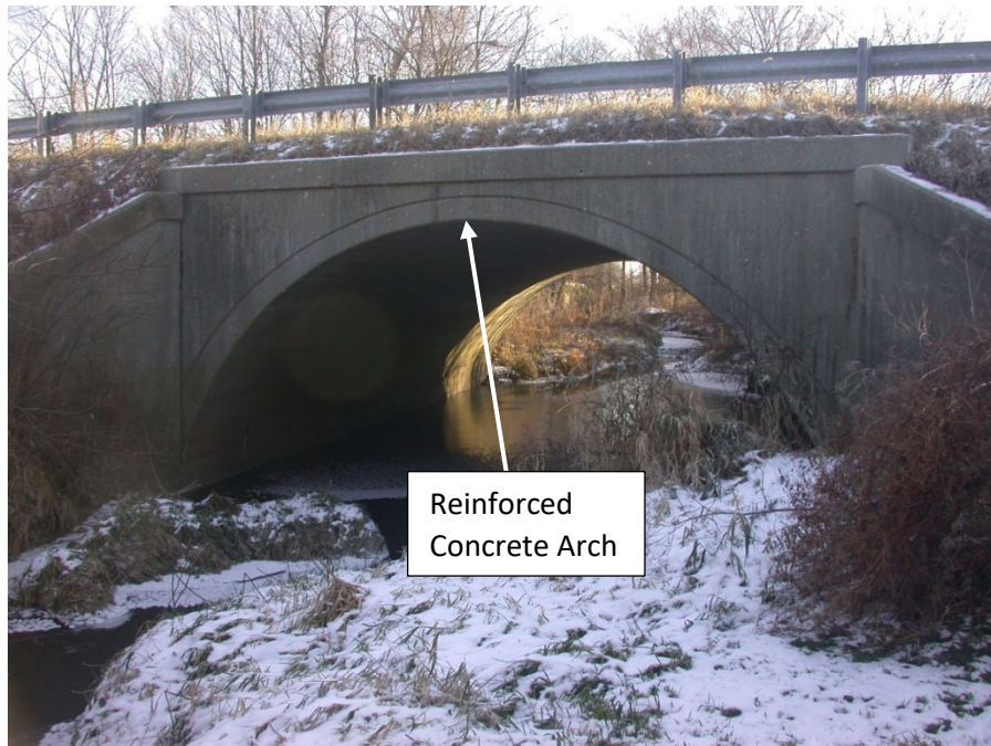
Reinforced Concrete Arch Bridge (Under Fill) with no cleaning or flushing activities required.
