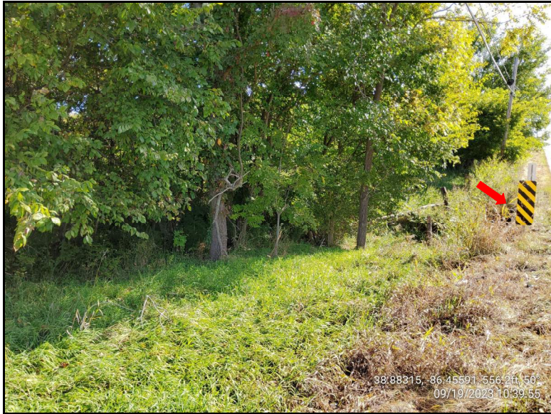
Photograph 53. Taken from SR 58 west of the CMP, facing northeast showing roadside vegetation and forested area north of CMP inlet. Red arrow indicates CMP.
