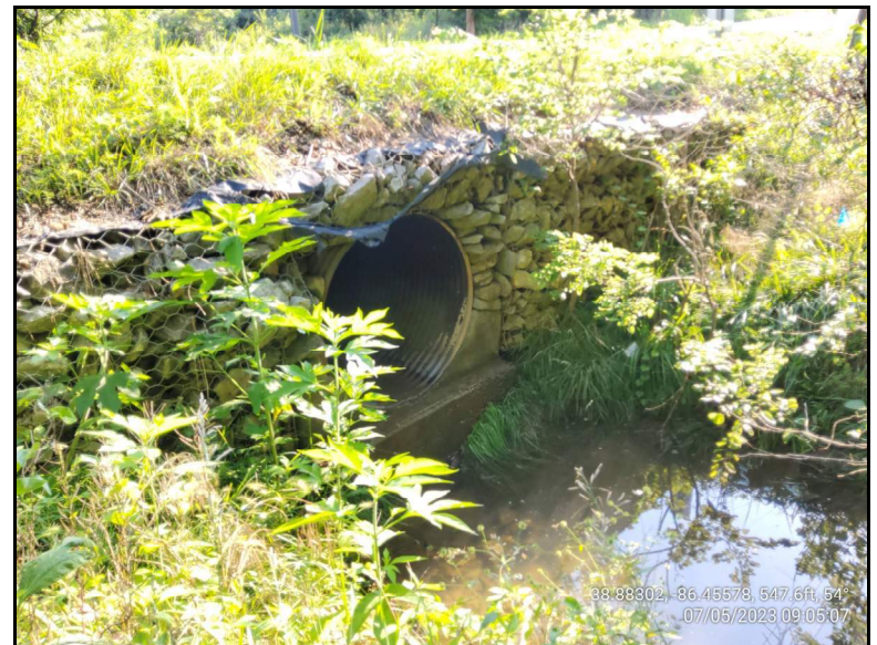
Photograph 36. Taken south of SR 58, facing northeast (upstream) in UNT to Leatherwood Creek showing the CMP outlet.
