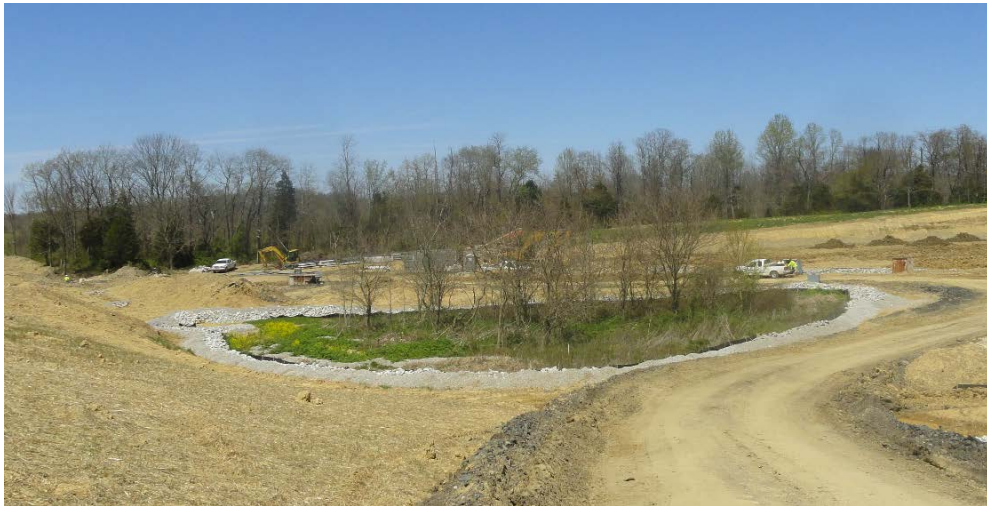
Rock ring protecting a very large karst feature on the U.S. 50 North Vernon Bypass Photo credit INDOT
