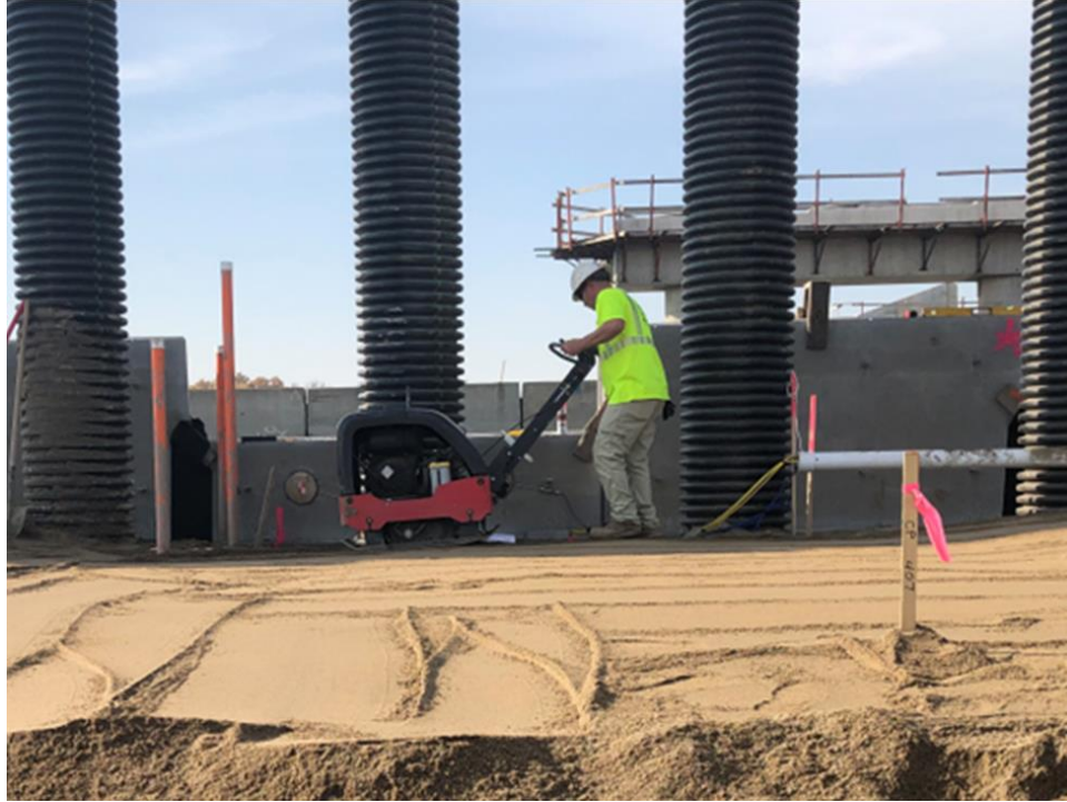
Figure 59. Typical vibratory plate compactor for compacting backfill within 3 ft of pre-cast panels
