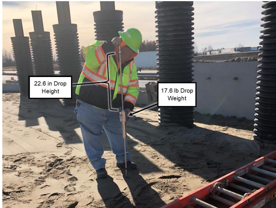
Figure 34. Conducting a dynamic cone penetration (DCP) test for acceptance testing of foundation soils and backfill compaction
