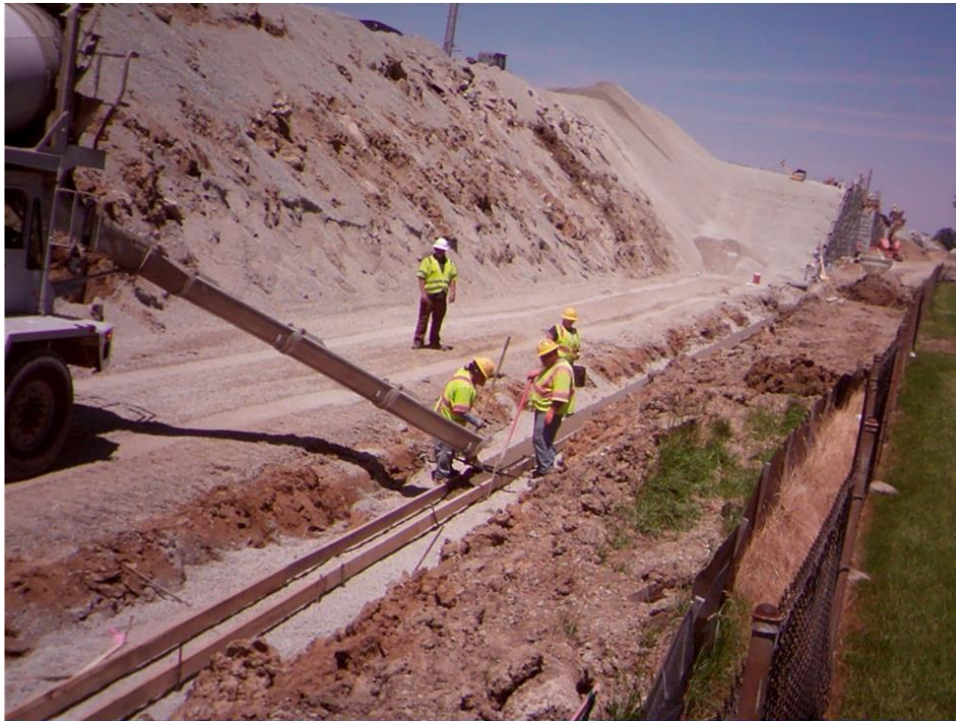
Figure 36. Typical MSE wall leveling pad construction operations that involve placing formwork and pouring concrete
