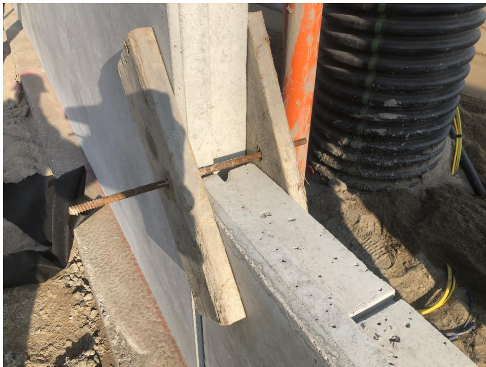
Figure 52. Example of adjacent pre-cast panels clamped together for maintaining alignment during construction
