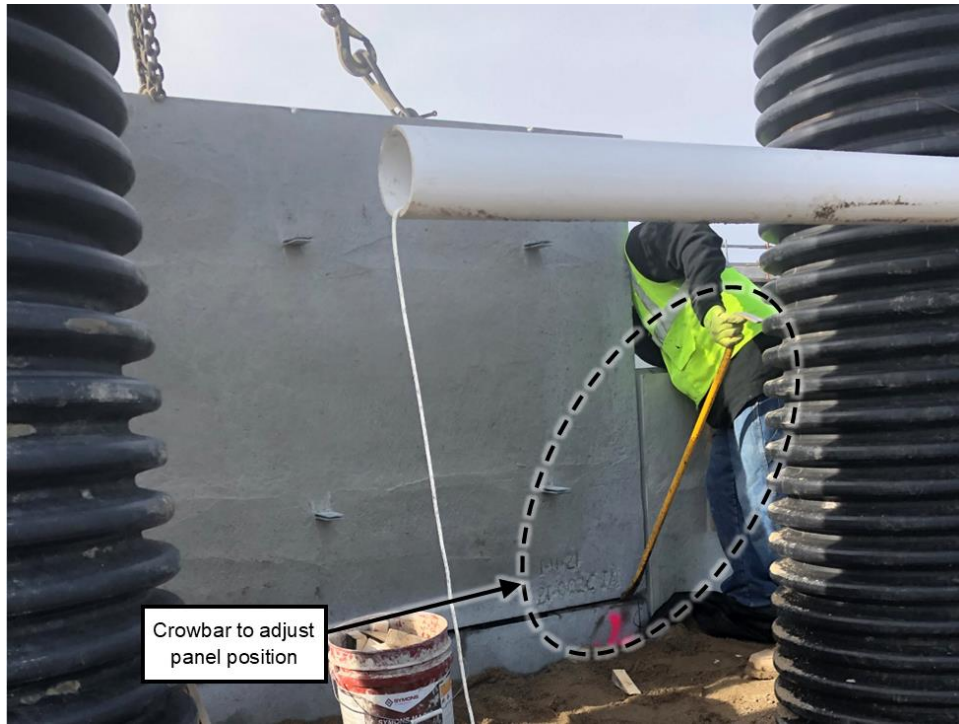
Figure 44. Using a crowbar from the backside of a pre-cast panel to adjust positioning
