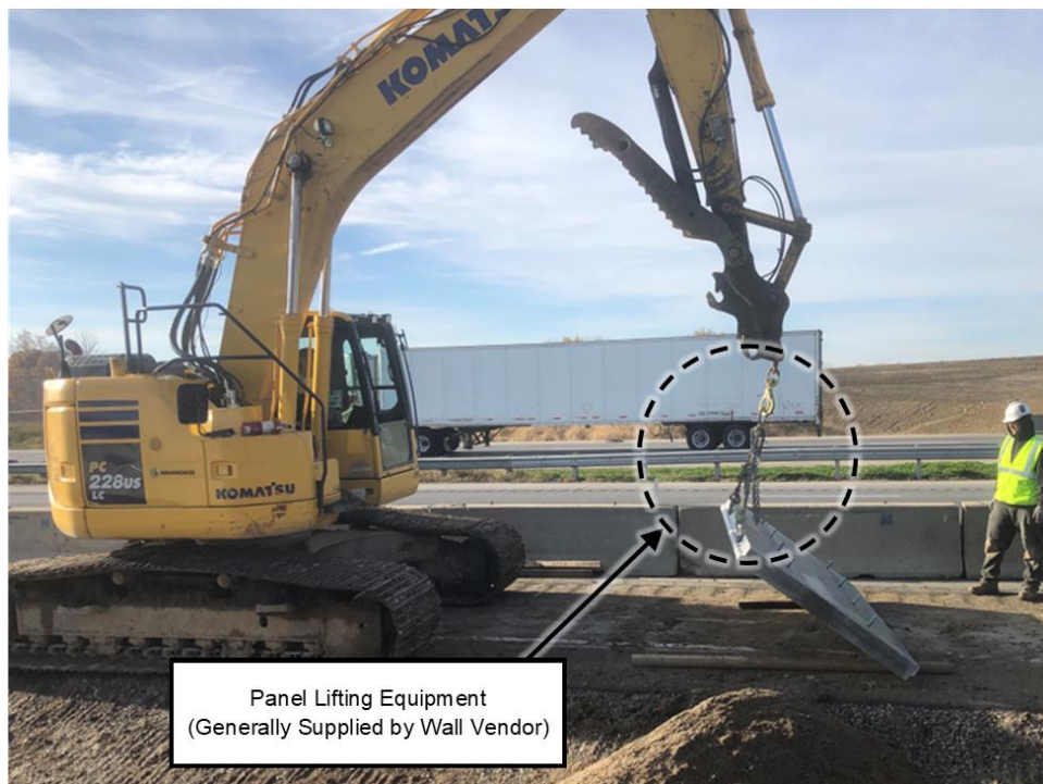
Figure 41. Typical pre-cast panel lifting and placement using MSE wall system vendor supplied panel lifting equipment and appropriate construction machinery
