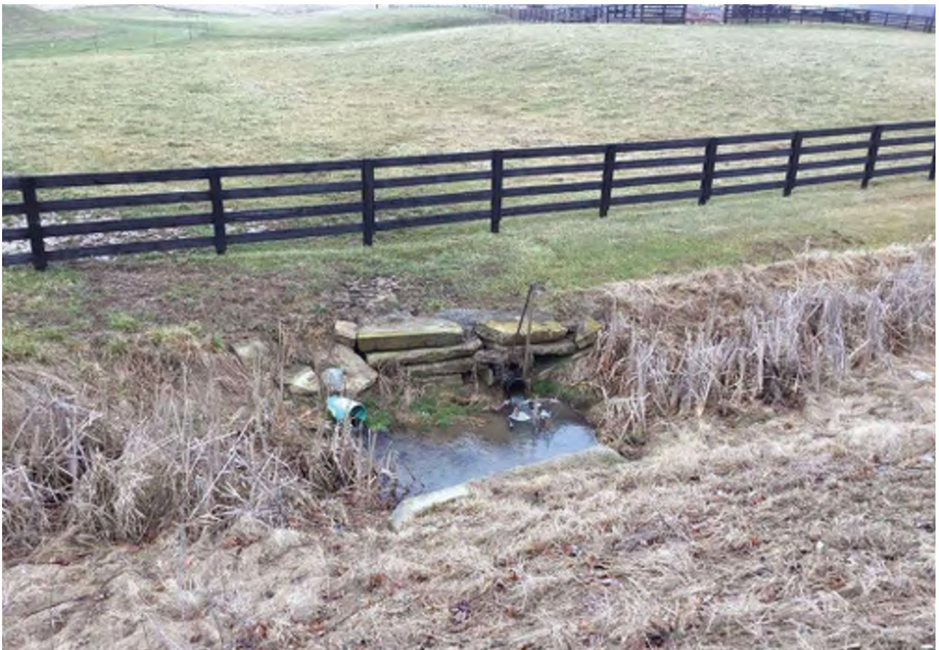
6 Looking northeast at the top of “Non-contributing” concrete headwall for drainage pipe running under SR 46, and stacked pieces of broken concrete as headwall to field drain pipe outlet.
