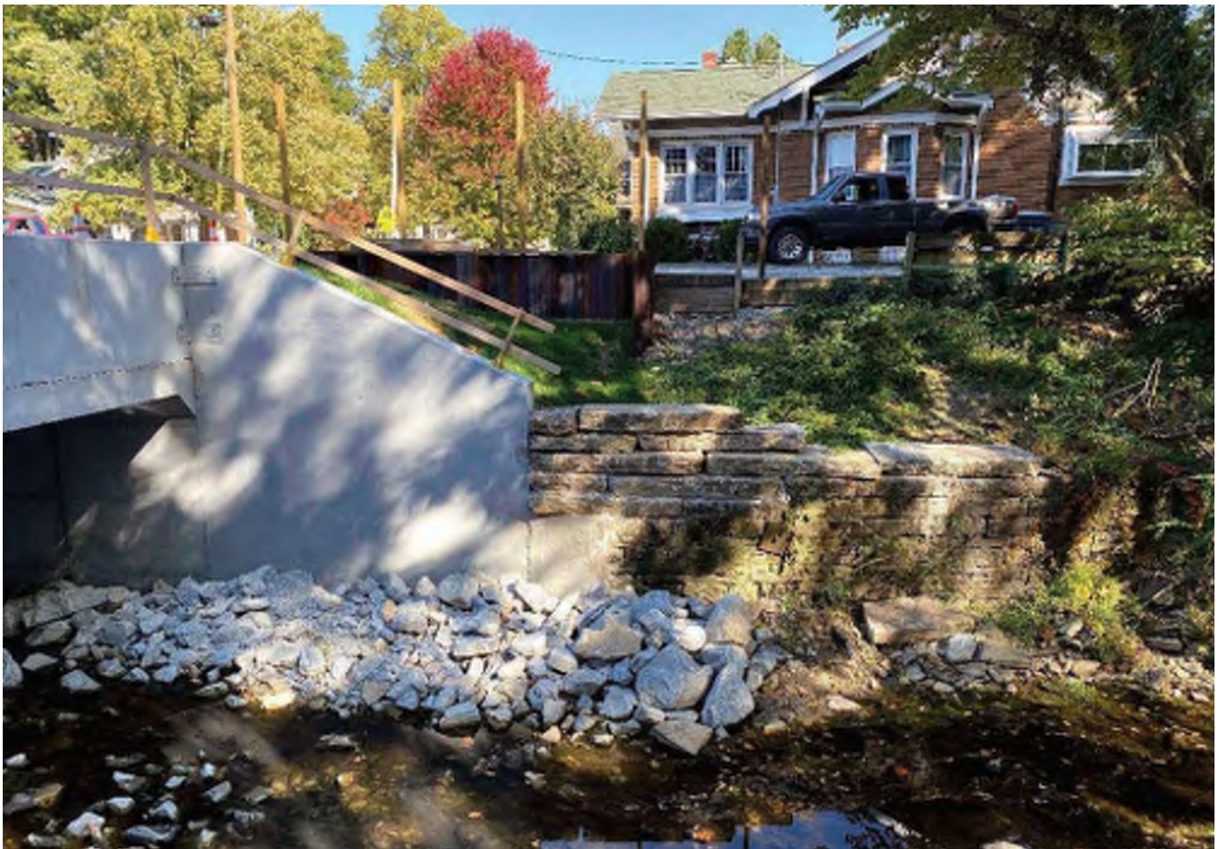
63. October 2020 photo looking east at new contemporary concrete bridge tying into original stone wing walls within the Greensburg Eastside Residential Historic District.
