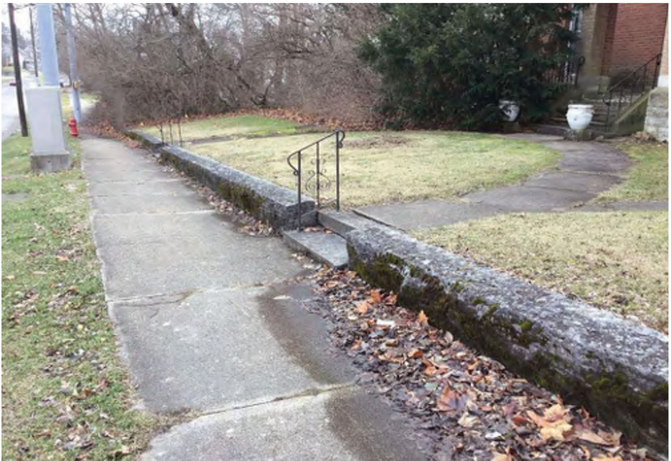
56 Looking southeast at the limestone wall and steps in front of the State Register-listed Charles Zoller House (NR-0308) property.
