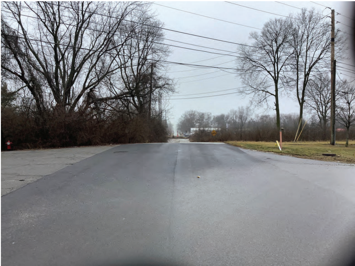
10. Looking N from S edge of project area on S CR 1050 E
