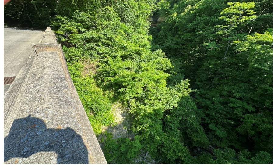
Photo 10: Facing north from the center of the bridge looking at the steep slopes and an erosional feature outside of the project area.
