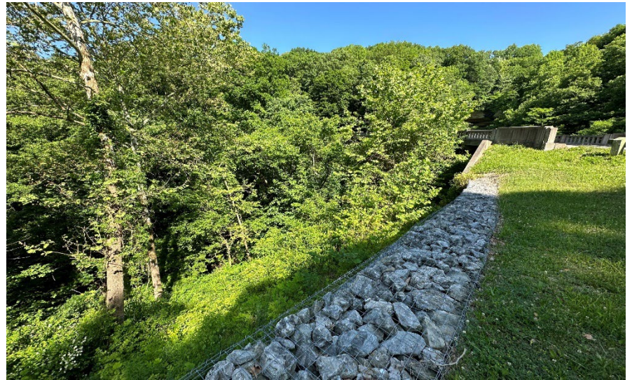
Photo 22: Facing north looking at the steep riprap lined slopes southeast of the bridge.
