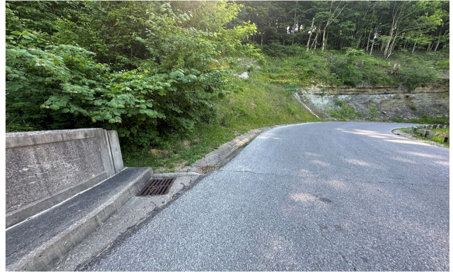
Photo 14: Facing east looking at a drain and a concrete roadside ditch (RSD) on the northeast side of bridge.
