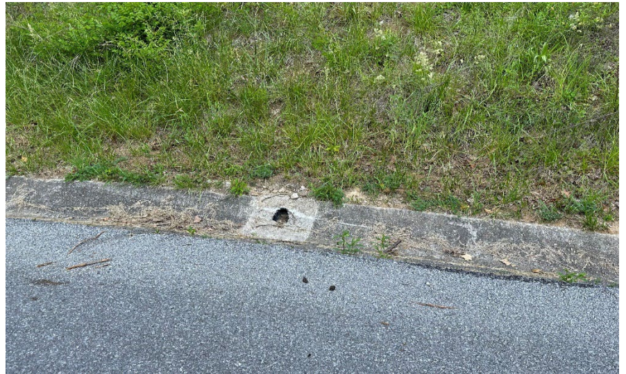
Photo 16: Facing east looking at a drainage feature on the north side of Park Road, east of the bridge.
