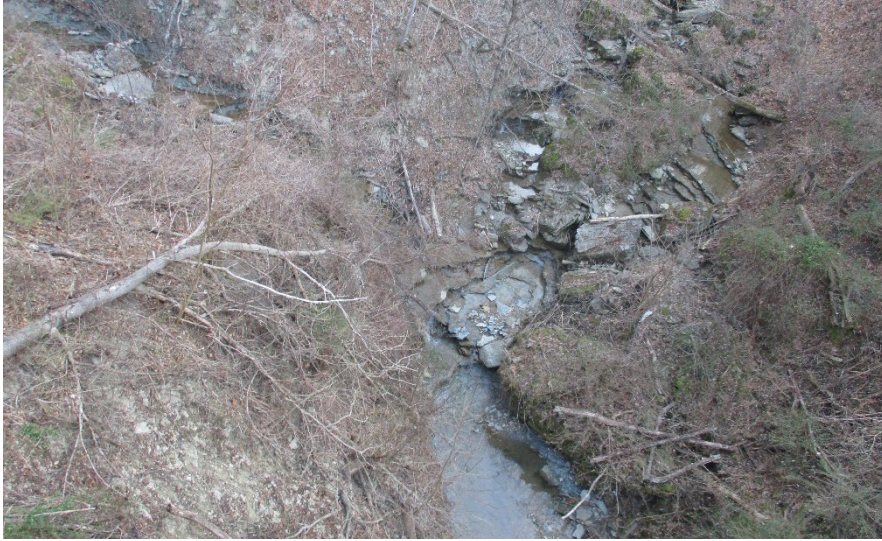
Photo 29: Facing northeast, looking down at Little Crooked Creek from the center of the bridge.
