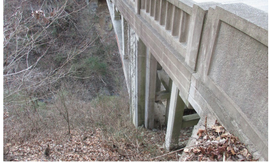
Photo 30: Facing northwest, looking down towards Little Crooked Creek from the southeast corner of the bridge.
