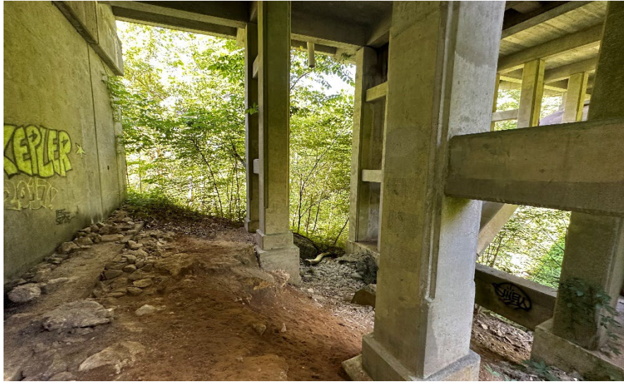
Photo 25: Facing south looking at the bridge abutment on the north side of the bridge.
