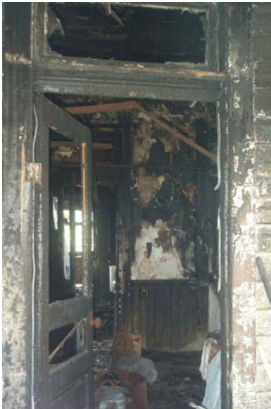
Gibson 30005-House, view east, detailed view of fire damage.
