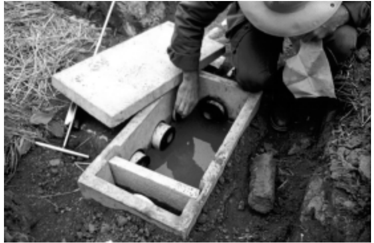
Figure 4-8. Distribution box with adjustable weir outlets
