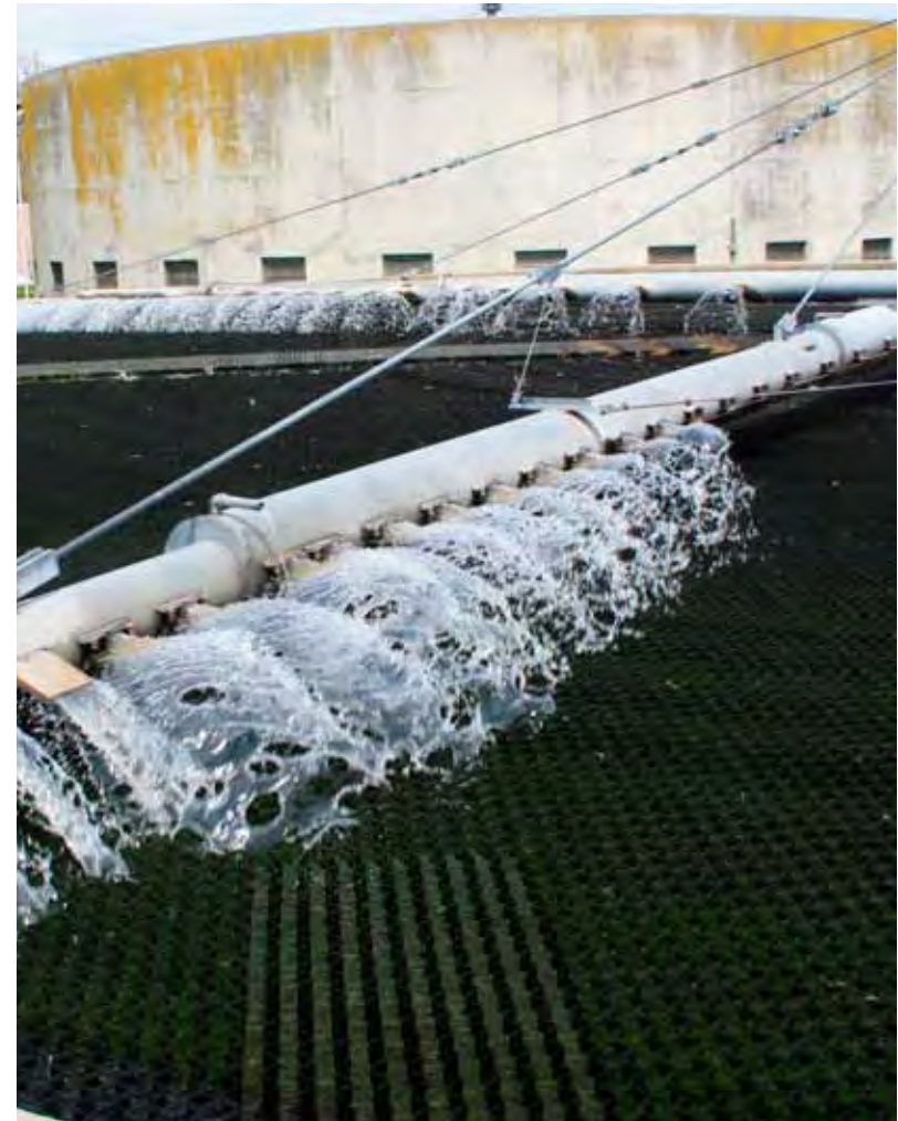
Wastewater Treatment Plant. Photo by Montgomery County Planning Commission, via Flickr, CC BY-SA 2.0 License.
