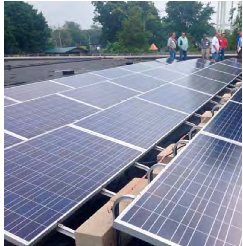
Rooftop solar panels at Porter County Career & Technical Center. Photo by Ty Warner.
