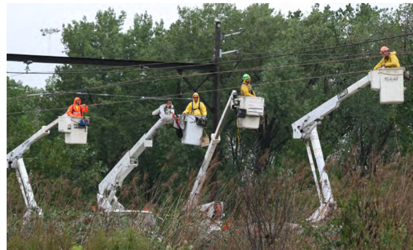
NICTD maintenance. NIRPC photo.
