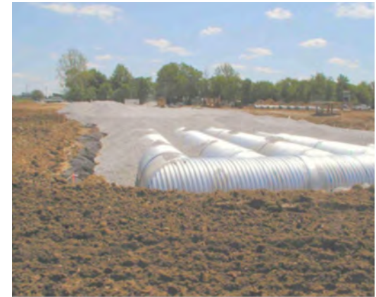
Subsurface detention/retention system.
