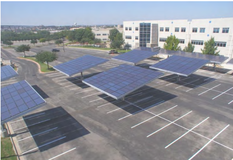
Photovoltaic panels in parking lot. Photo from web.
