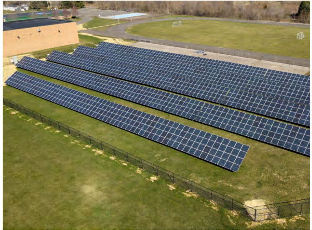
North Liberty Elementary Solar Farm (Source: Veregy)
